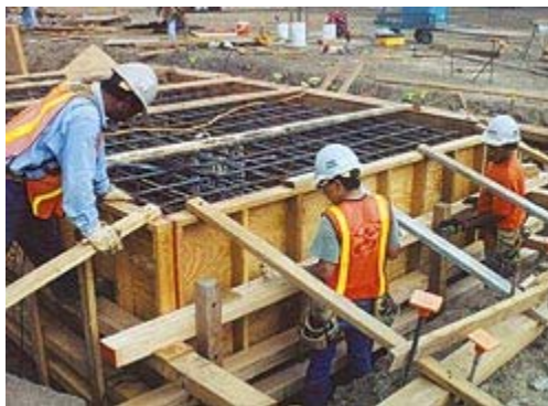
Working on a form at the Wal-Mart/Sam's Club construction site off Keeaumoku Street, are members of Hawaii Carpenters Union, Local 745. Photo courtesy Hawaii Carpenters Union.
