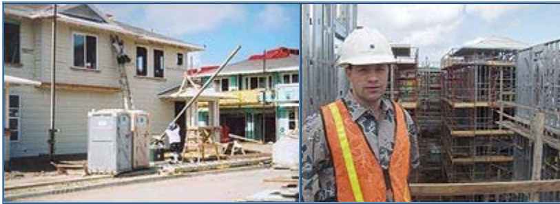
Stanford Carr Development is creating the Cottages and the Villas in Hawaii Kai. Above, Rick Papa, project manager for Stanford Carr Development, oversees construction of the Colony — a four-story luxury condominium at the Peninsula in Hawaii Kai.
